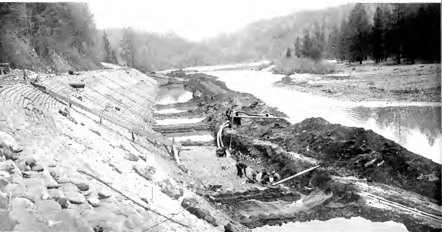
Workmen placing strip of wire and rock mattress in river bed at foot of riprap protected slope
